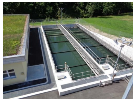
Sedimentationsbecken PAK-Stufe (links Filter)
