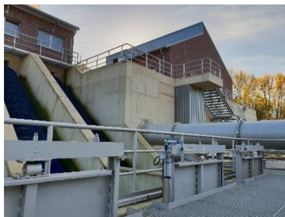
Fig. 10: Installation d'ozonation Aix-la-Chapelle/Soers (source: WVER)
